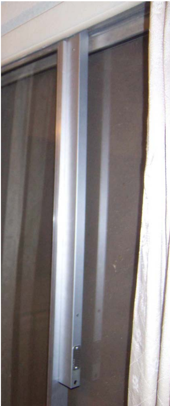
Cable closer mounted on door
